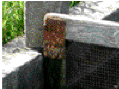
Outflow screen held in place by cement block could be knocked over
