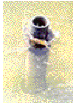
The slots in this vertical stand-pipe provide a barrier for fish and debris
