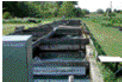
Hérons must be able to wade or perch close to the water to fish effectively. The side of this raceway is too high from the water for the heron to reach the fish
